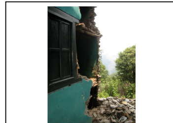
..... but the rear view shows extensive damage
